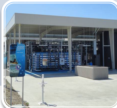
Potable Water Reuse
