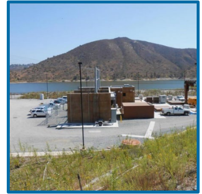
Lake Hodges Energy & Pumped Storage Projects $208 million
