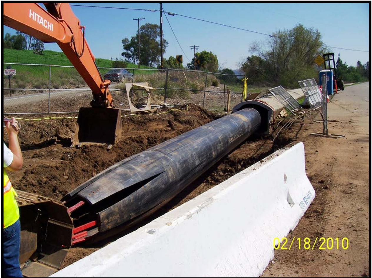
Figure 32: Inserting HDPE pipe into the MW bench, 2010. A portion of the flume was demolished to establish an insertion point.
