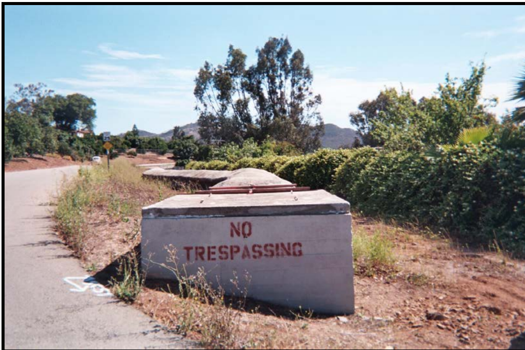
Figure 8: Typical concrete box at end of flume, where it is connected to an underground siphon.
