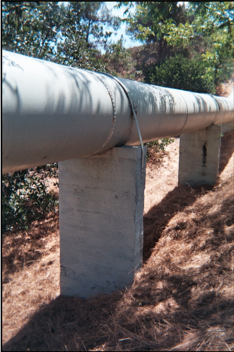
Figure 12: Typical above-ground steel pipe supports of Twin Oaks Siphon across shallow ravines.
