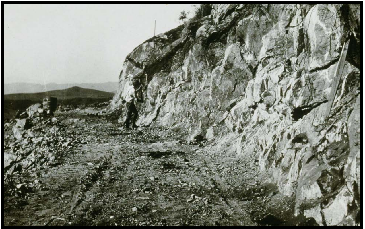
Figure 16: The first step in constructing the flume was to build the road bed.
