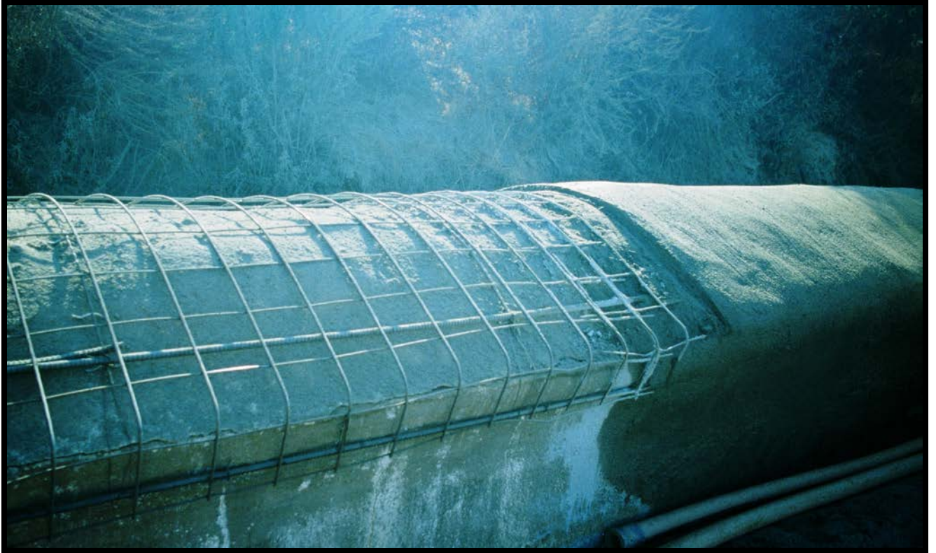
Figure 31: In the 1980s a second flume cover with steel rebar reinforcement was placed on top of the first.
