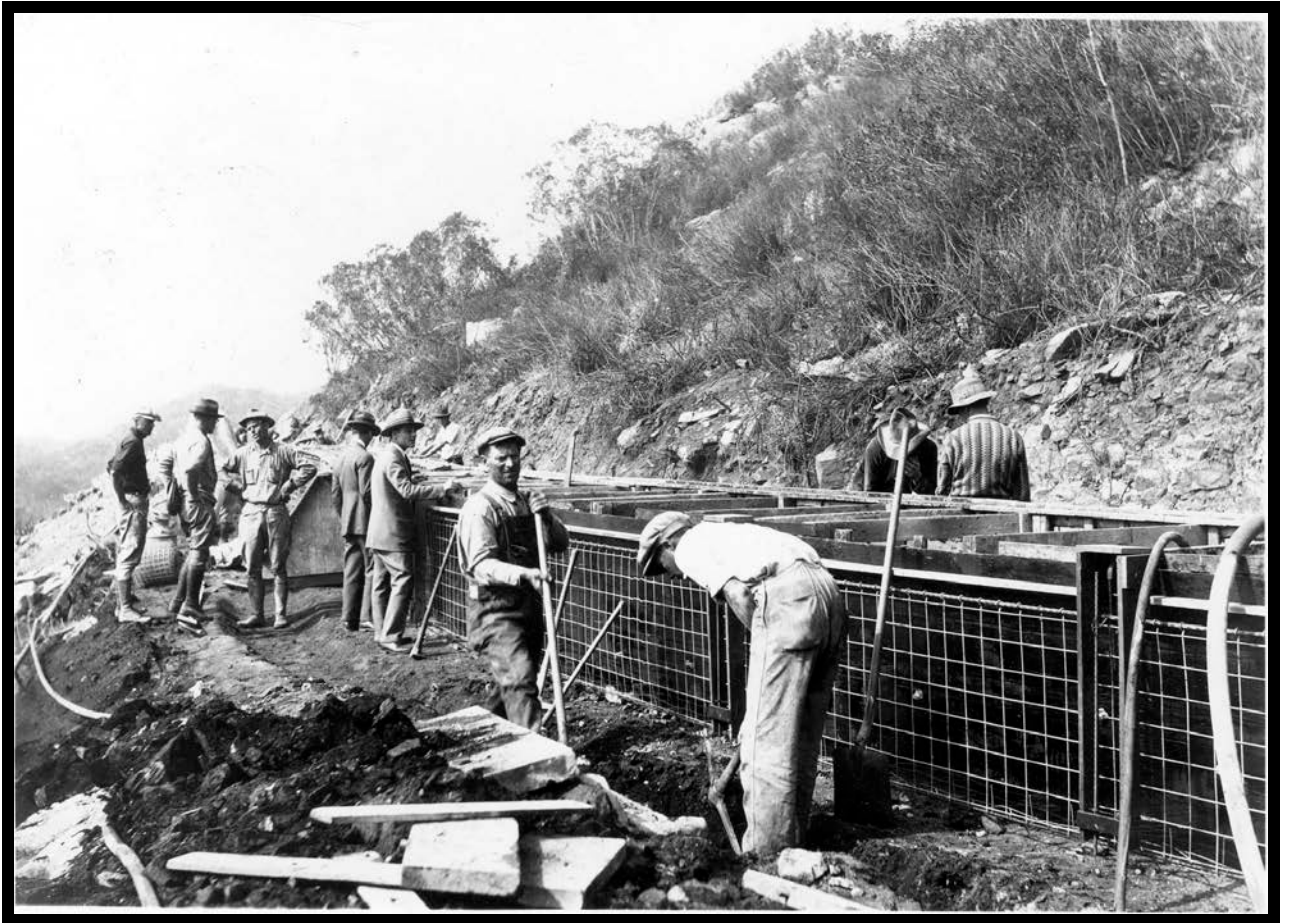
Figure 17: Gunite bench flume construction 1926. Note the welded wire mesh held in place by wooden forms (Courtesy Vista Irrigation District).
