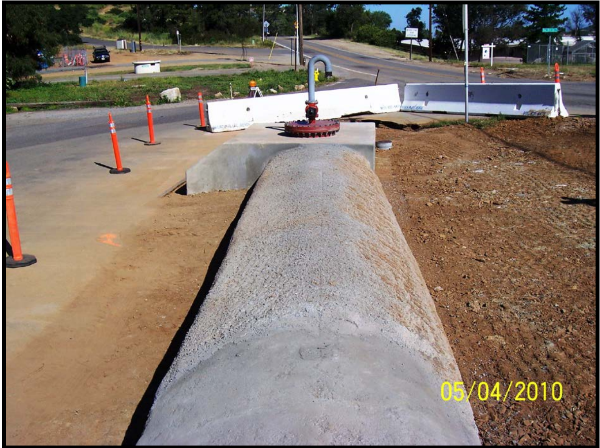
Figure 33: Repaired section of MW Bench after completion of the HDPE pipe insertion project.
