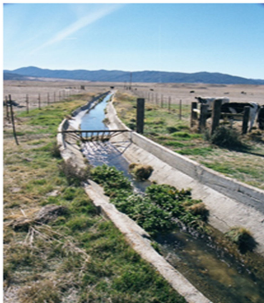
Figure 6: Weeds growing on the ditch downstream of the trash rack.
